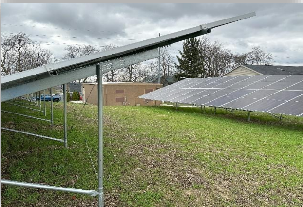
Figure 17: The 97-kW solar PV array at the Middletown central office is sized to provide 100% of the power needed at the CO over the course of a year making it altafiber's first net zero central office.
