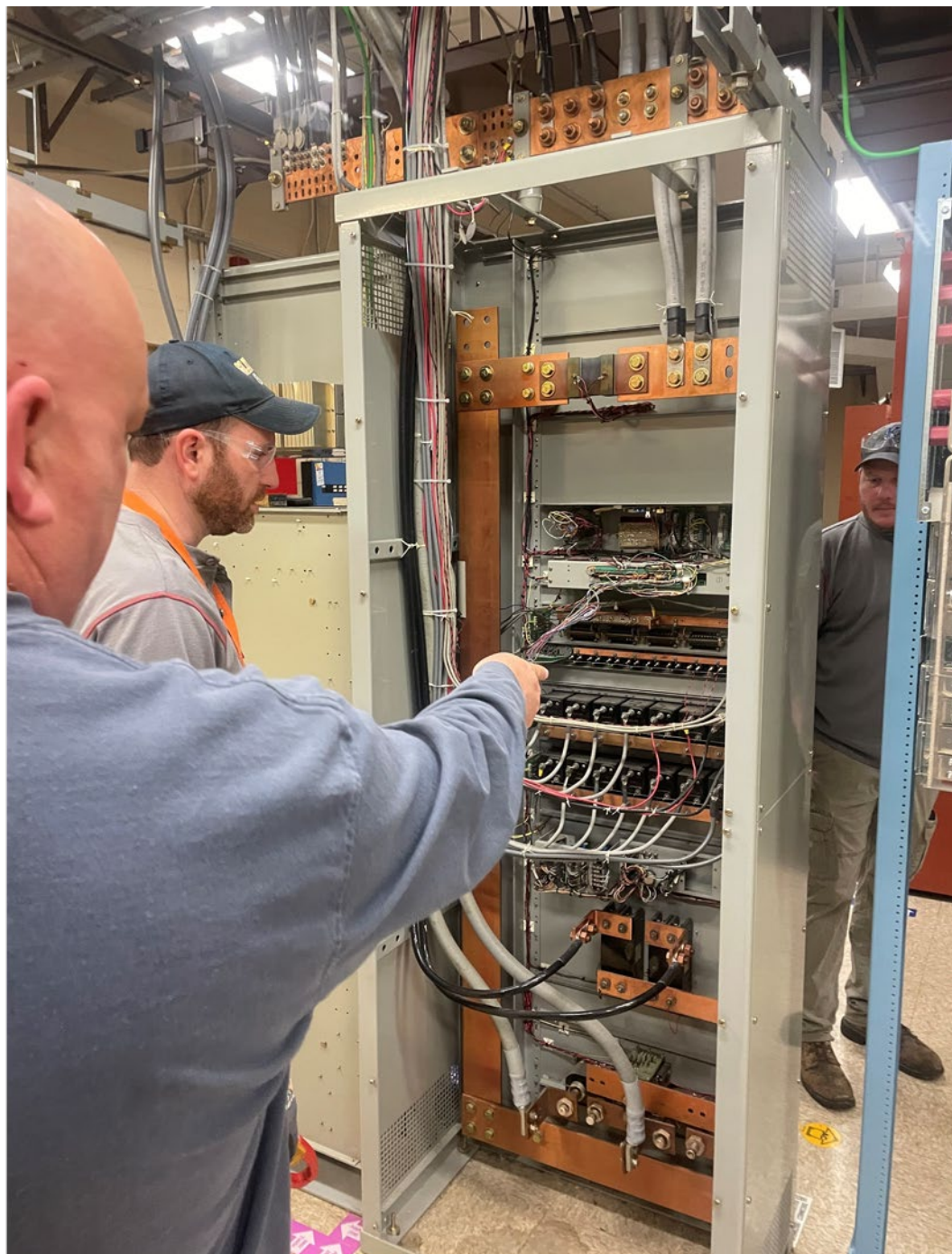
Network Operations Center employees turn down a voice switch in Cincinnati.
